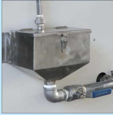
手動入藥水缸 Manual chemical feeding tank
